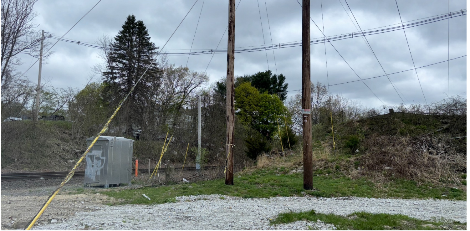
Photo #3: View of Pole 12 (Z126W #15) on the WS1 Line, located within the 100-ft Buffer Zone to BVW. Facing North
