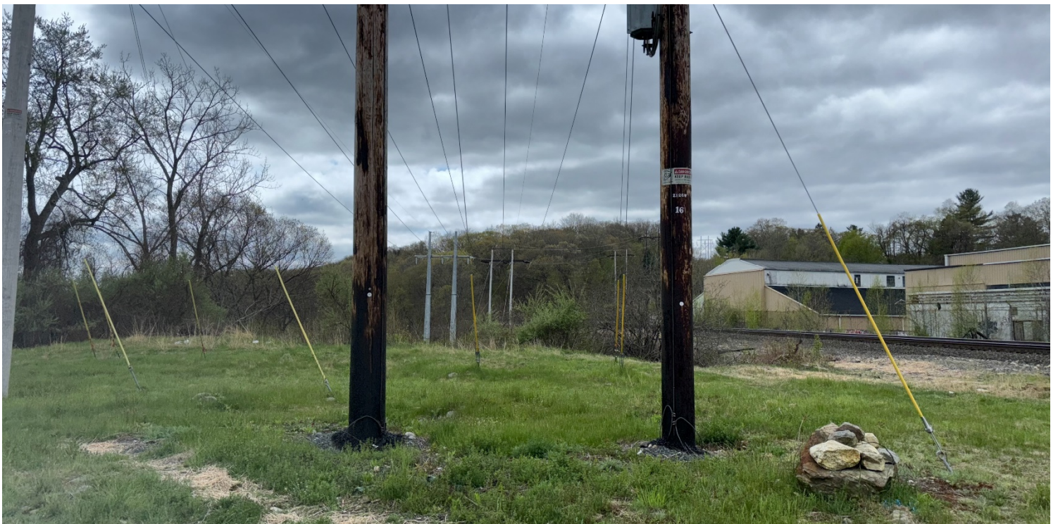
Photo #2: View of Pole 11 (Z126W #16) on the WS1 Line located within the 100-ft Buffer Zone to Bordering Vegetated Wetlands (BVW). Facing south.
